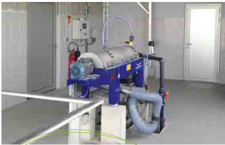
Cosmetics Sludge dewatering
